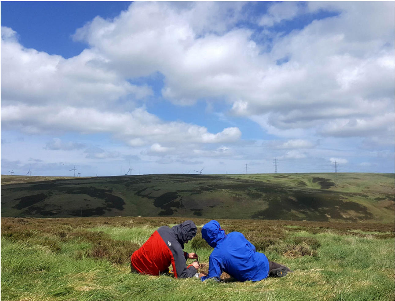
Tony Swan and Tim Taylor installing a SWIGS system near Whiteadder Reservoir in East Lothian
